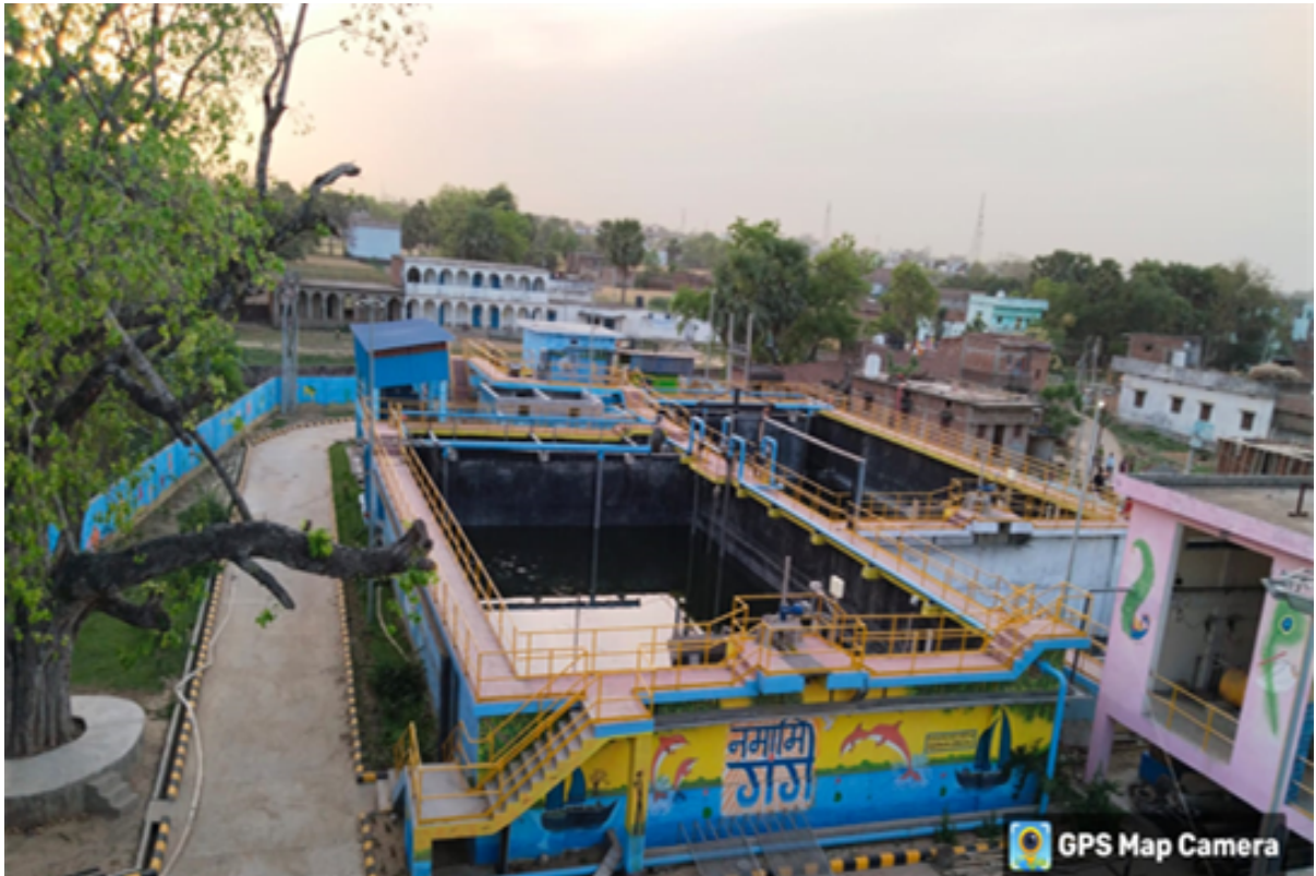
6.50 MLD STP at Patna-Maner
