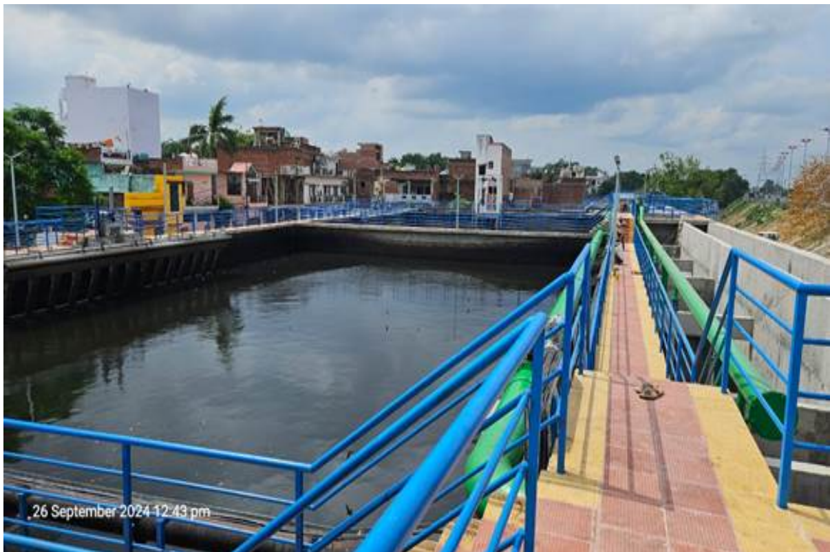
39 MLD STP at Lucknow
