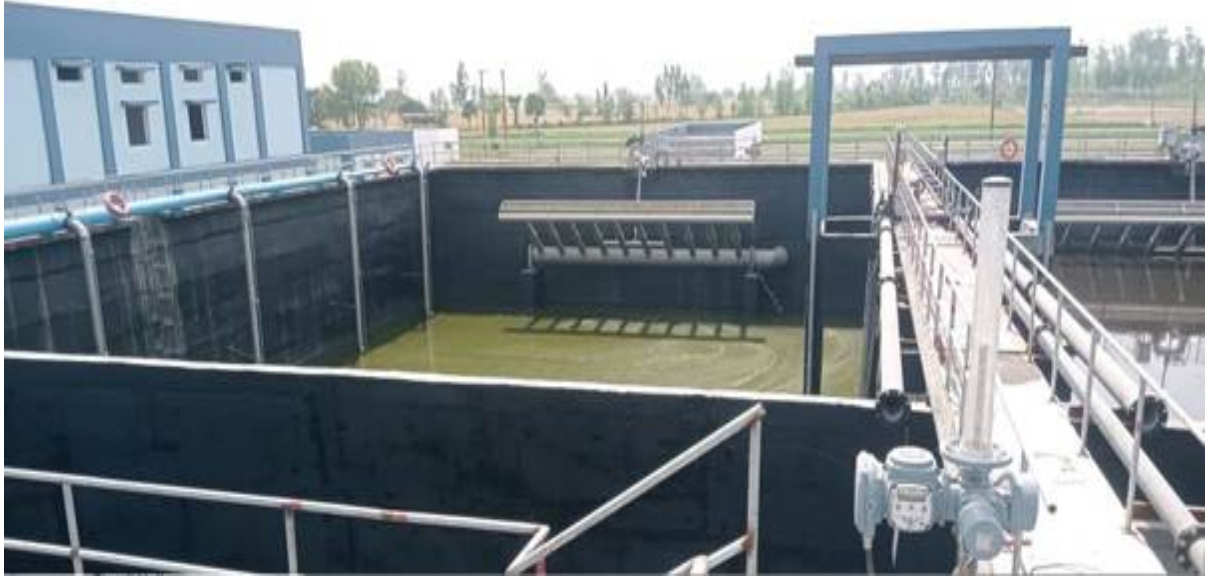
15 MLD STP at Kairana
