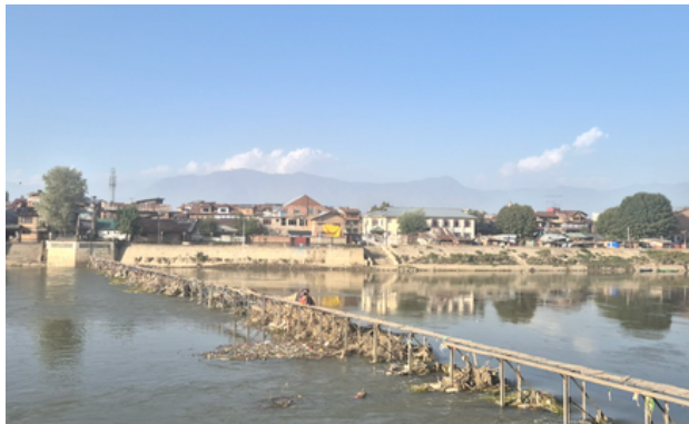
Weir maintained by Irrigation and Flood Control Department, acting as a solid-waste trap.
